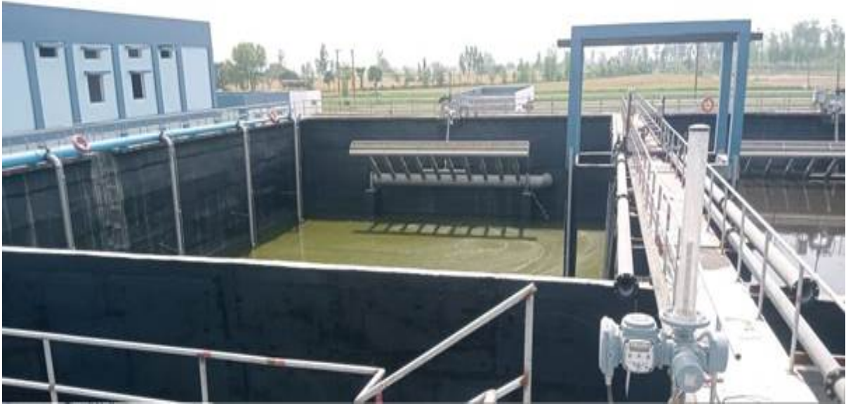
15 MLD STP at Kairana
