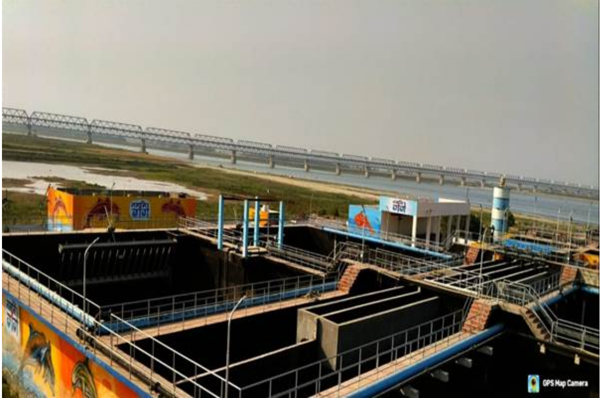
25 MLD STP at Patna-Danapur
