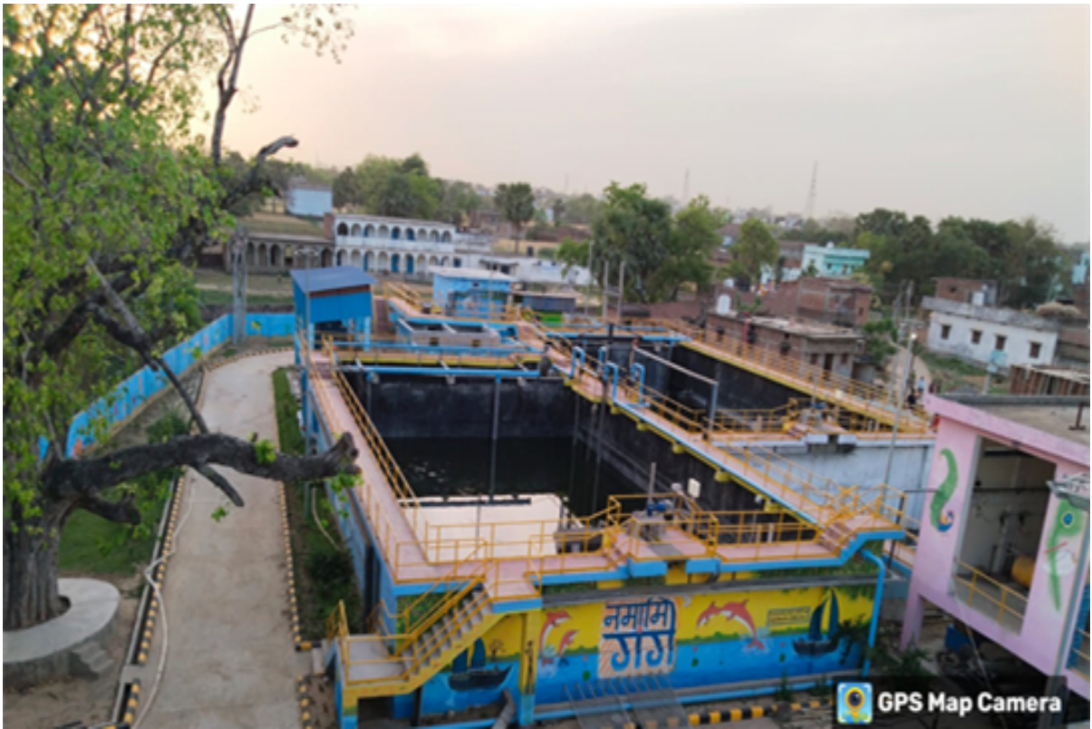
6.50 MLD STP at Patna-Maner
